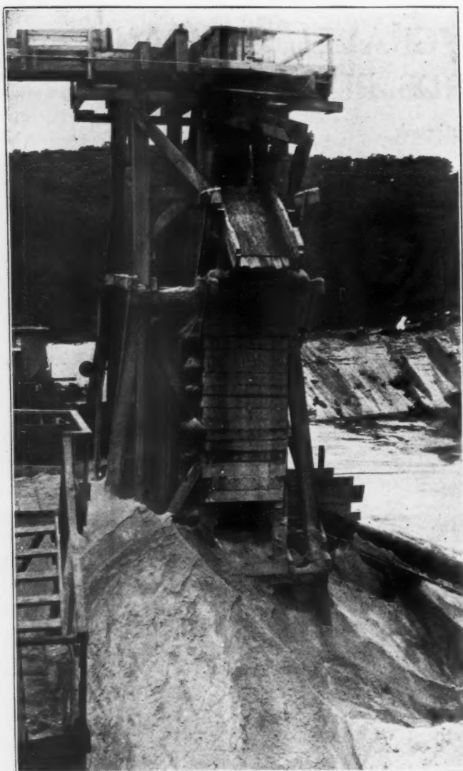
One of the Wooden Towers to Which the Sand Is Elevated and Then Discharged to the Storage Pile
